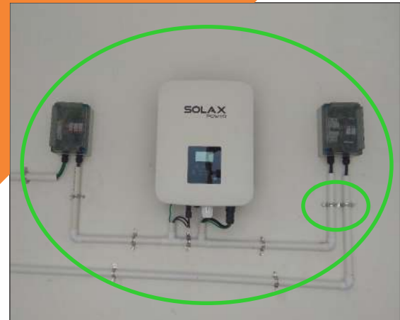
Neat and clean electrical work with UPVC conduit pipe. Use of screw for longer durability.
