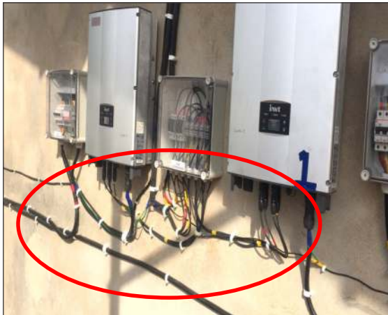
Open wiring may cause problem. Weather may effect open wiring.
