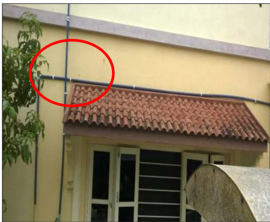
Black or blue conduit pipes are sometimes not esthetic.
